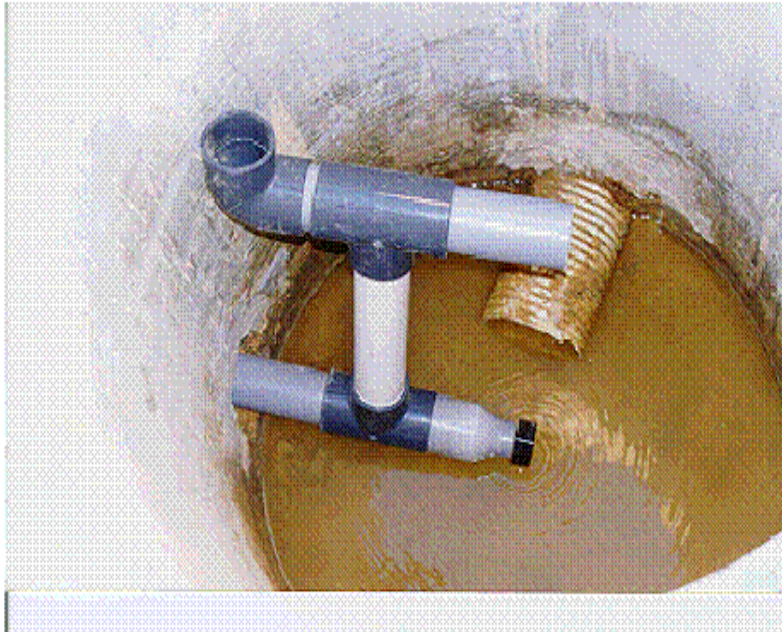
Figure 8. Water table control device
