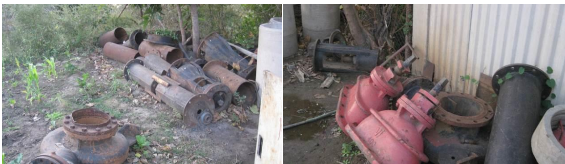
Figure 13 Part of the remains of the sand abstraction system equipment at Tsvovani
