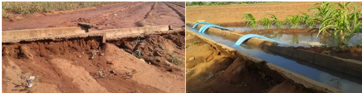
Figure 10. Eroded canal embankments in Vimbanayi and Mutorahuku schemes
