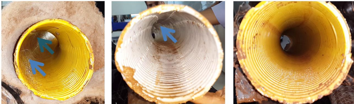
Figure 7. Visual inspection for root growth after excavation of the drain pipes with a geotextile (left), no envelope (middle) and Hydroluis® combination (right).
