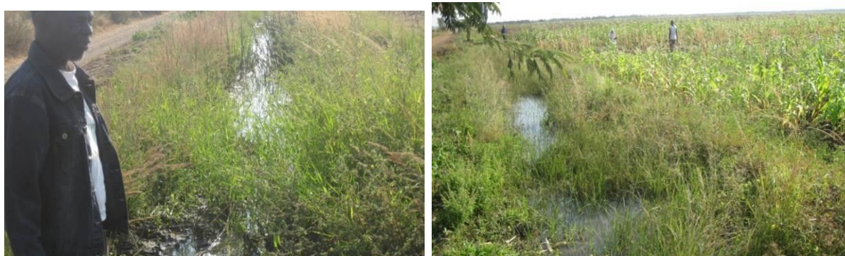
Figure 9. Shallow and grass choked canals at Tsvovani irrigation scheme
