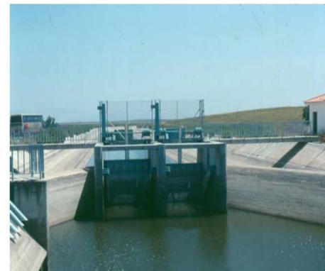
Spain: Cabral Project, SCADA
