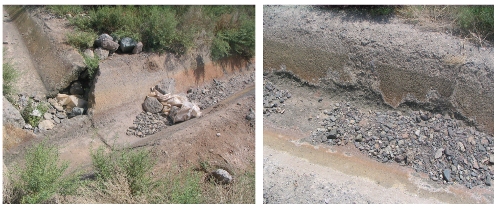
Fig. 2. Damage to lined irrigation channels.
