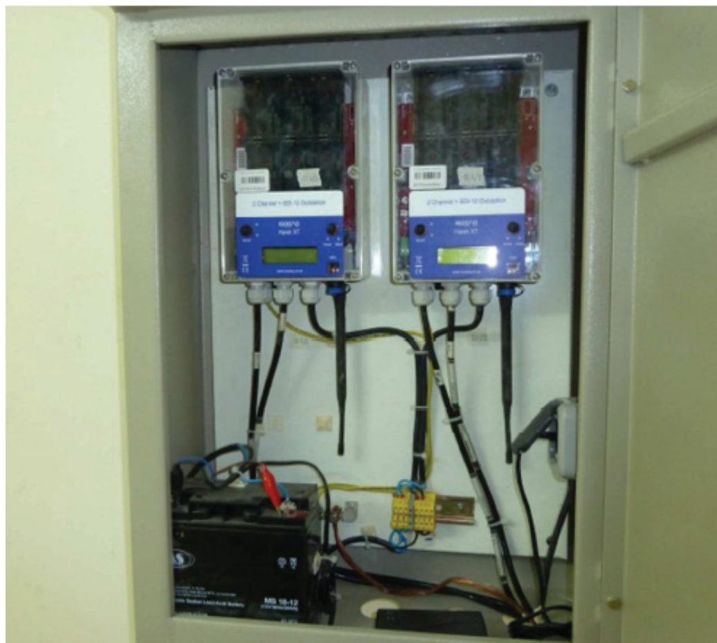
Fig. 7. Logging devices at a Parshall Flume gauging station
