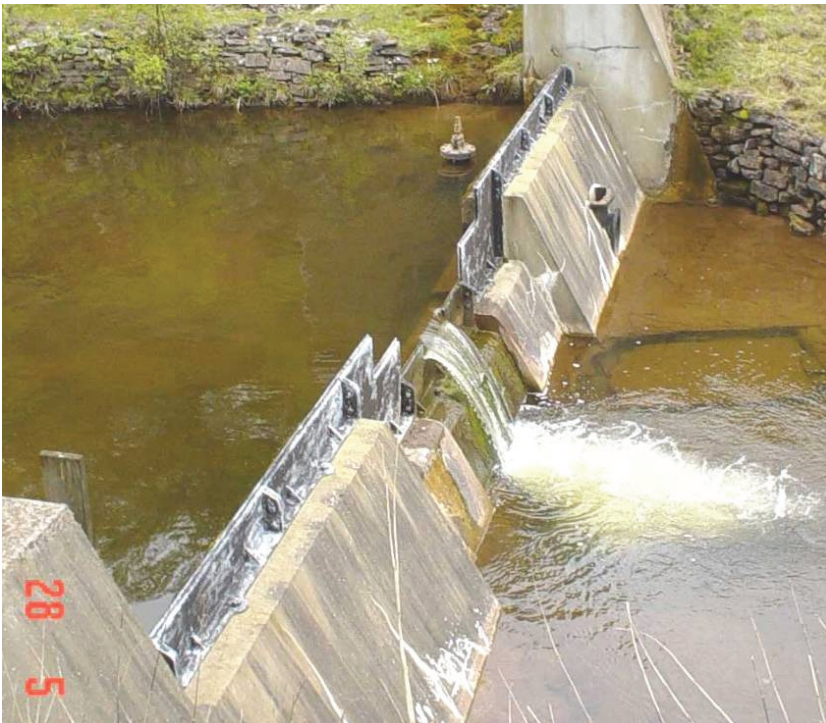
Fig. 4. Example of thin plate weir gauging structure
