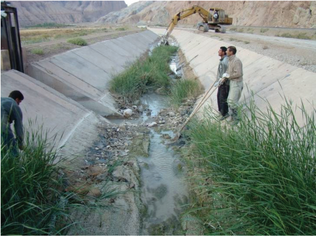
Fig. 11. The problem of silt accumulation and vegetation growth
