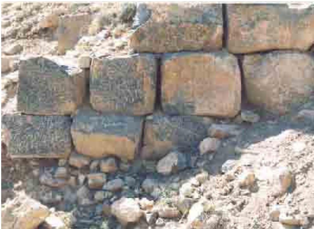
Figure 14. The remaining of a stone retaining wall close to Didegan dam.
