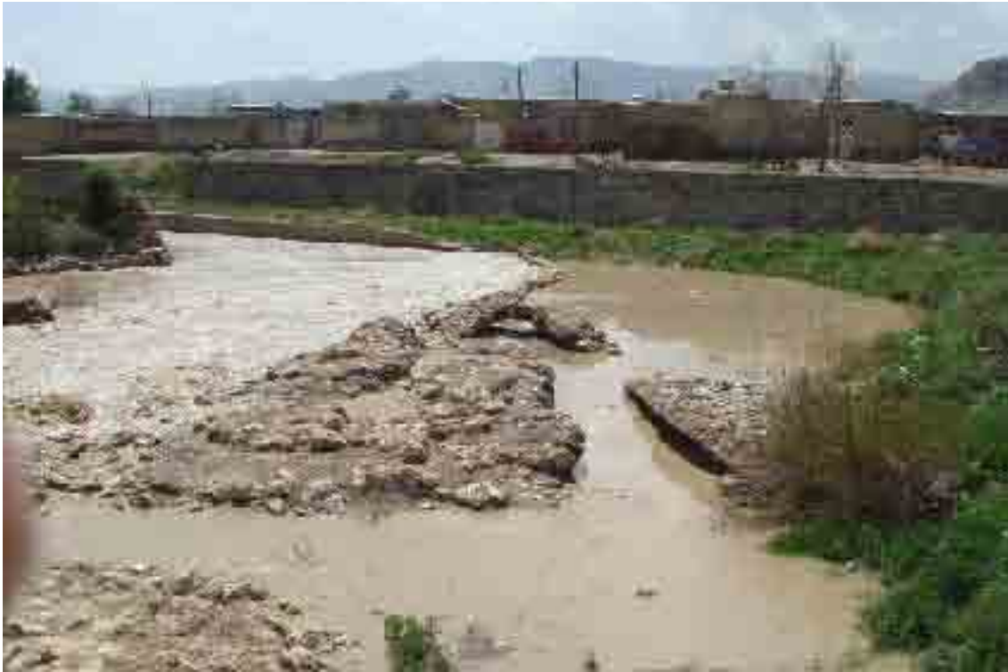
Figure (5). The remains of sediment flushing conduit of Amir weir (right)
