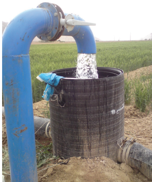
Fig. 2. Hydroflume intake from polyethylene barrel
