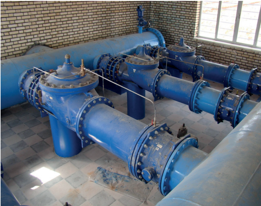
Fig. 3. Flow Control Valve Room
